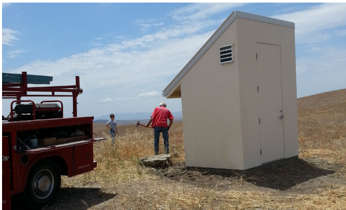
Figure 2.34.3. Installation of the surface hut at TRAM. Solar panels will be mounted on the south-facing roof. The door is 8 ft tall to allow access for installation of borehole equipment.
